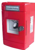
Centralized control BCCP unit for fire safety start / firefighter stop / pollution ventilation, at the reference level near each vehicle access.
