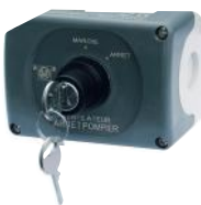
BAPA firefighter stop, at the reference level near each vehicle access.
