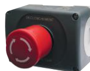
BREA reset unit, inside the car park.
